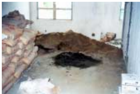
Figure 3.5 Left over mortar becomes waste
