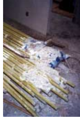
Figure 3.11 Lost of plaster while applying
