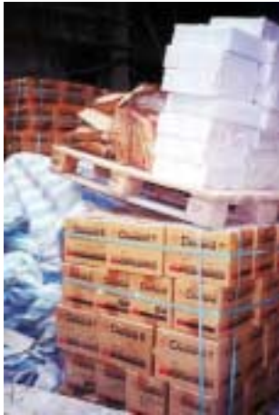
Figure 3.12 Improper stacking of blocks
