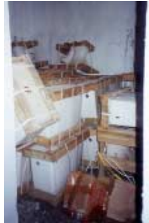
Figure 3.13 Damage of sanitary fitments
