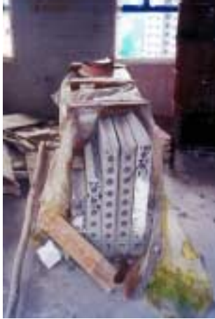
Figure 3.9 Damage of dry wall panels
