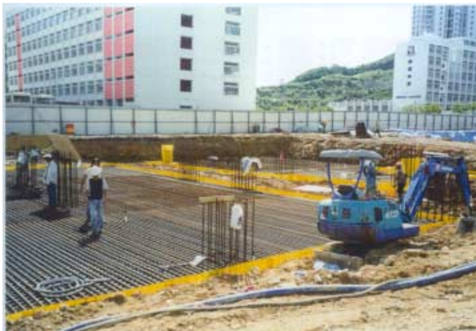
Figure 4.17 Backfill around pile caps about 150mm from the top level of Pecaform
