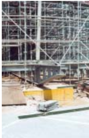
Left page: (top) General view of the pavilion under construction. (Middle) Prefabricated modules. (Bottom) Detail facade.
